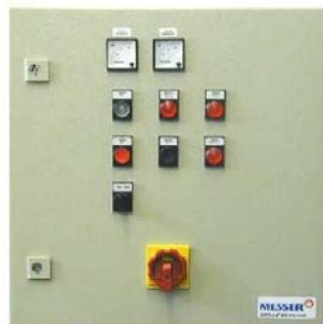
Control panel for monitoring heating torches
